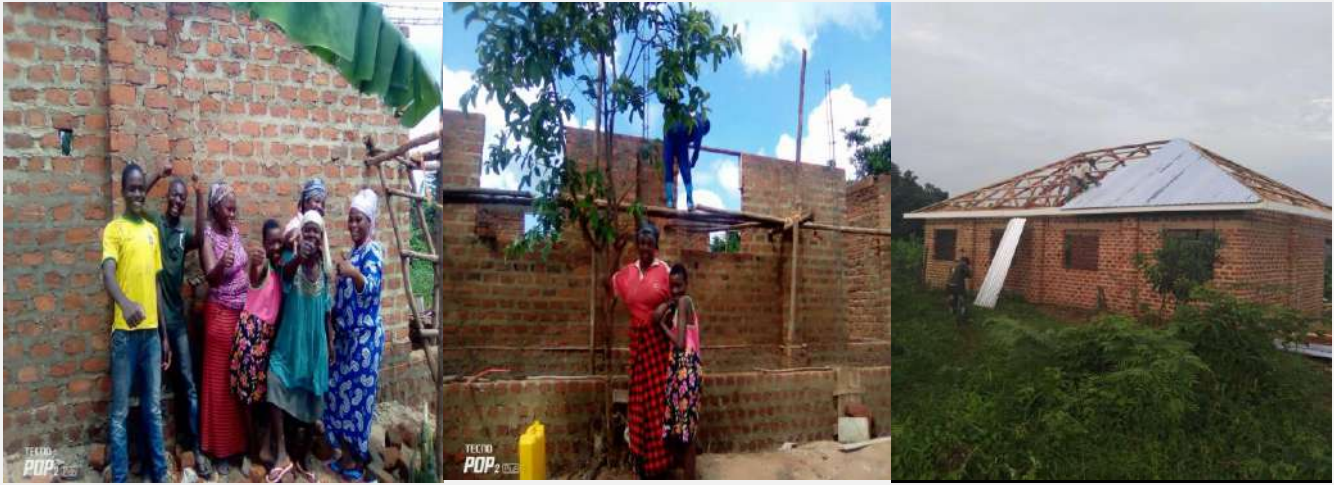
Smile of the Child Project children and Wangari women standing in front of the unfinished building; and the roofing of the building.
